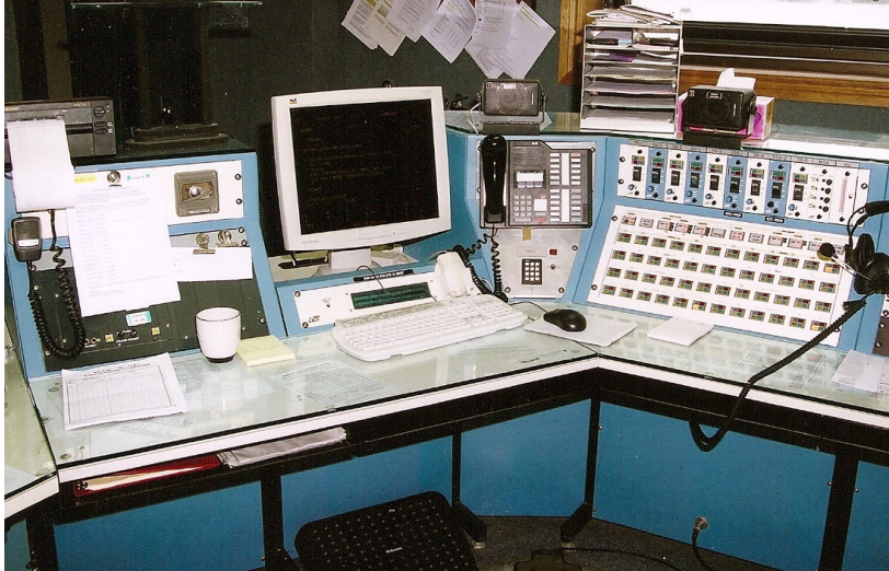
Close-up of one of the VHF consoles
