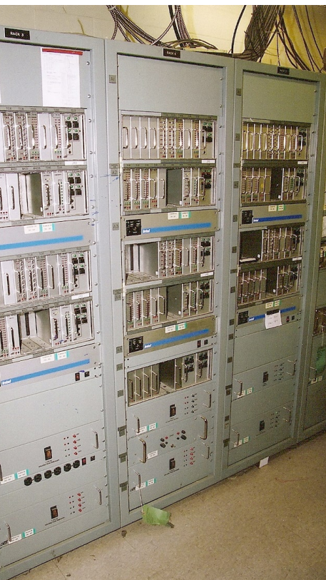
Remote telephone switching unit
