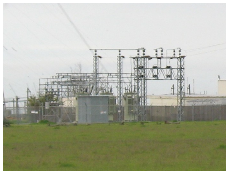
Figure 8 - VOA Dixon power substation.
