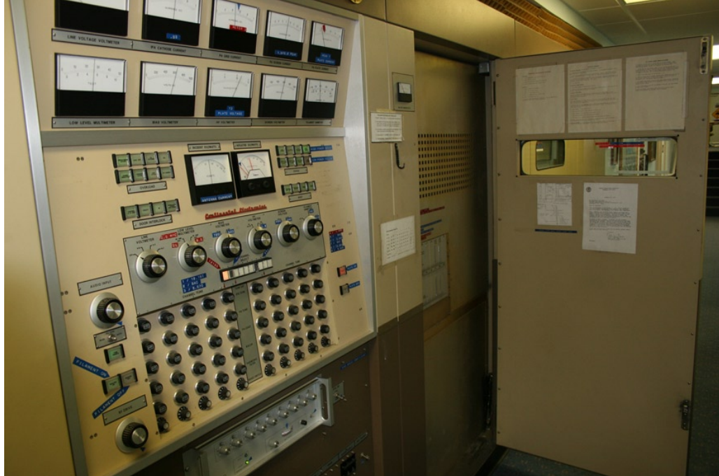
Transmitter #4 at WWCR from Continental Electronics pumps out 100 kW. New or used transmitters are still expensive buy, ship and operate. Care to pick up the electric tab at WWCR for a month? You can “borrow” this transmitter for as little as $15 for 4.5 minutes. (Photo by Cameron Keel courtesy WWCR)
