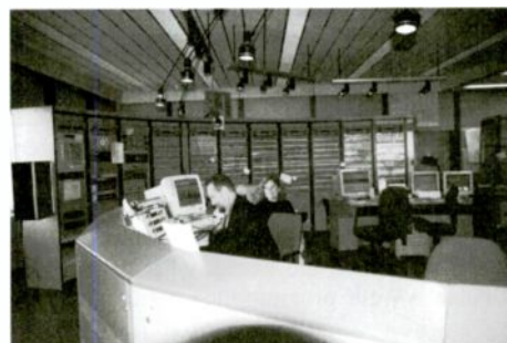
The master control room at the Cologne broadcast center, courtesy M Guha
