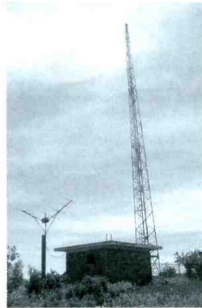
"V" shaped antennas at many longwave sites are for a separate 75 MHz marker beacon.
