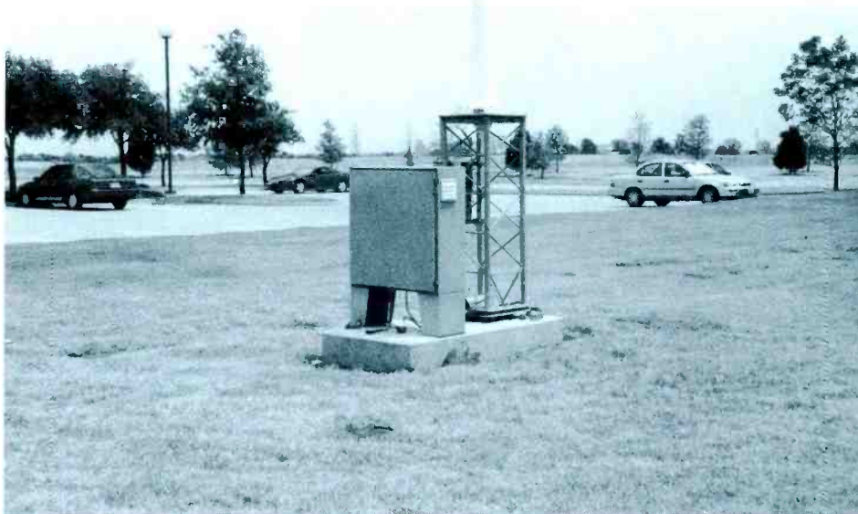
Closeup view of the base of the 1680 kHz arrival information TIS station at DFW Airport. The box contains the actual transmitter plus the antenna tuning unit.
