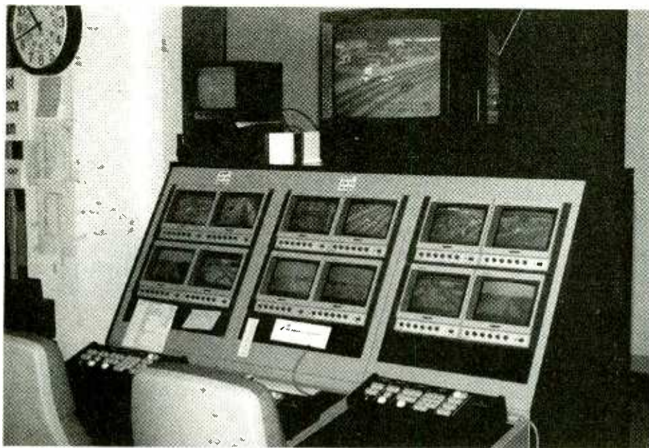
Closed circuit TV control console at Texas Dept of Transportation's Traffic Management Center.
