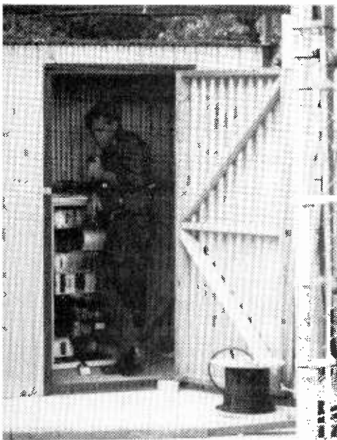
A Coast Guard technician repairs the high level site at Signal Mountain, Tennessee.
