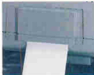
All cable plugs are neatly covered with plastic shrouds
