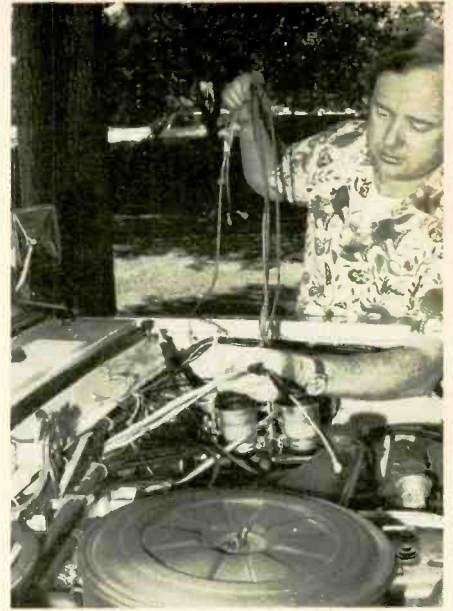
The wiring harness should be carefully pulled through the hole in the firewall so no slack is left inside the cab.
