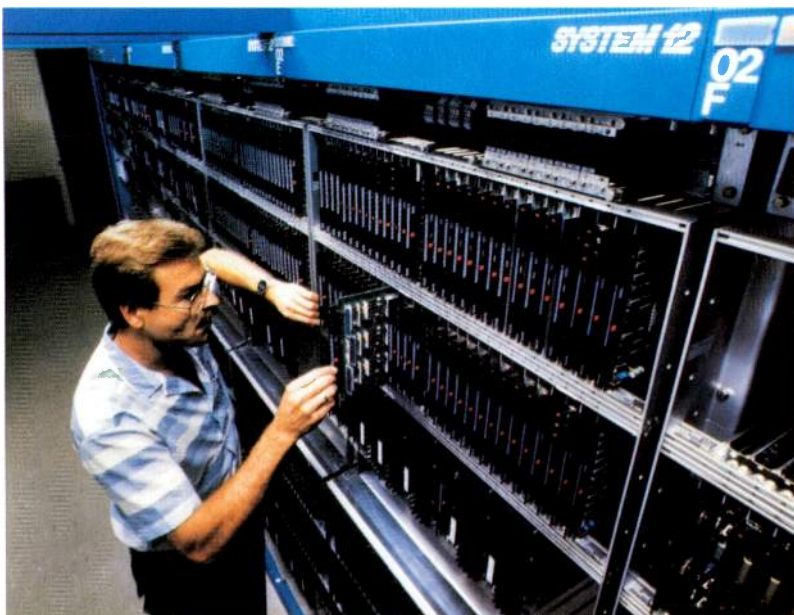
View of a typical System 12 exchange with the cabinet doors removed.
