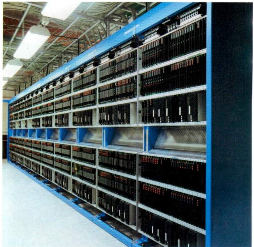
View of the large 3800-trunk System 12 toll exchange with the cabinet doors removed.
