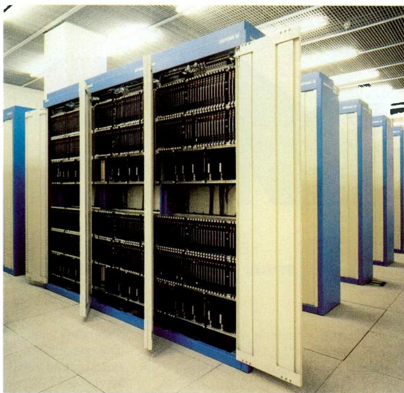
System 12 exchange equipment in the 10 000-line Salamanca exchange in Spain.
