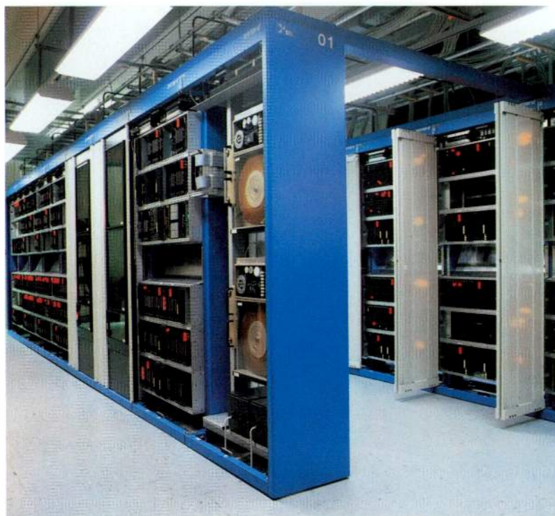
Large local System 12 exchange installed in Wuppertal for the Deutsche Bundespost.
