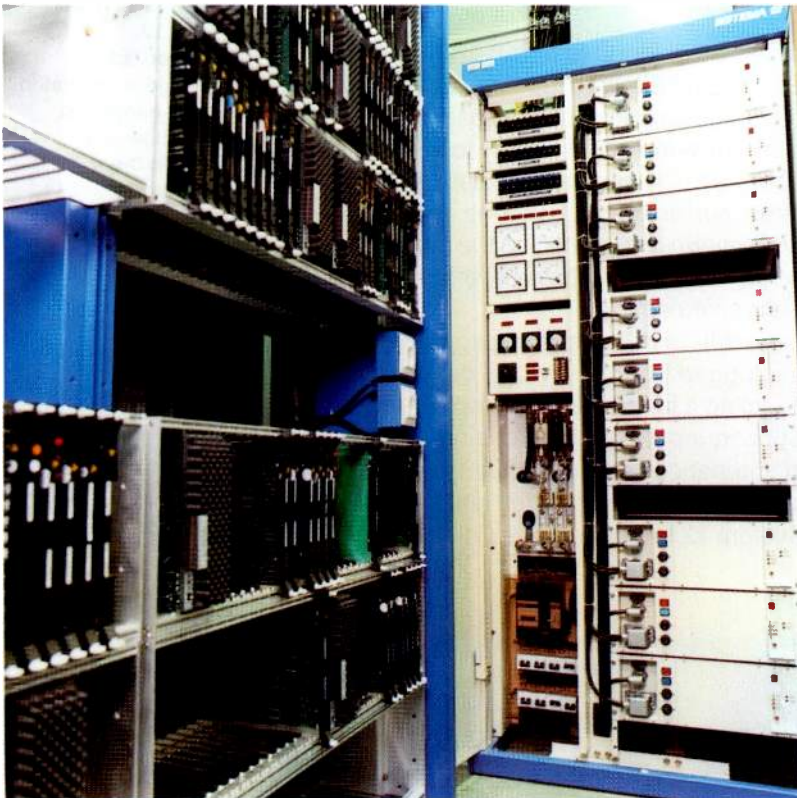
Modular power plant integrated into a System 12 rack.
