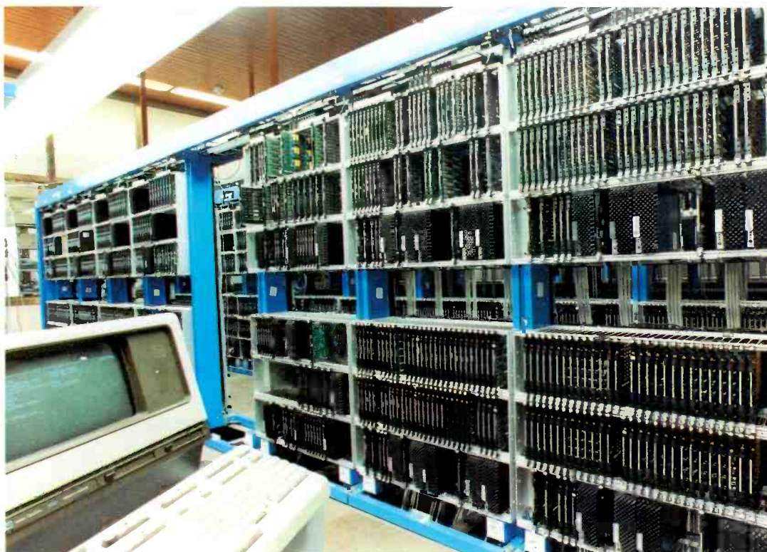
The System 12 Digital Exchange room at Acilia.
