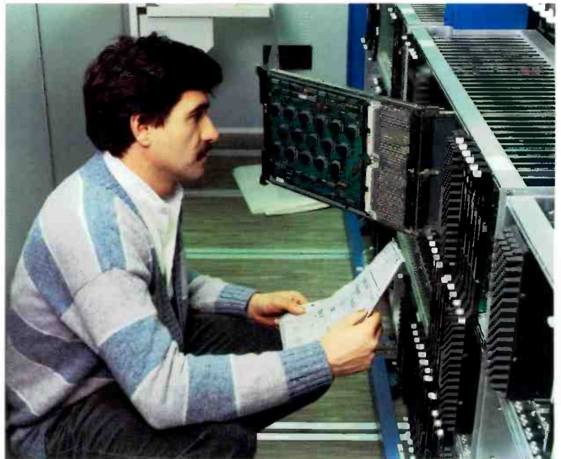
Maintenance of the System 12 containerized exchange is facilitated by wide gangways which allow easy access to the equipment.
