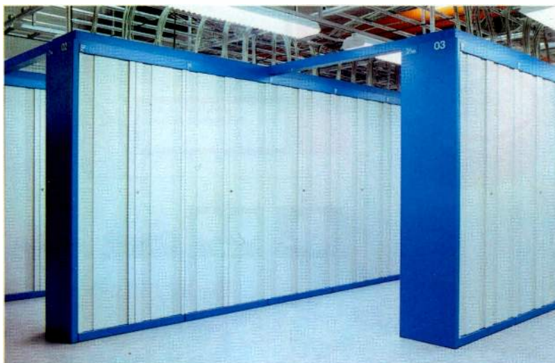
System 12 large toll exchange installed in Stuttgart for the Deutsche Bundespost.
