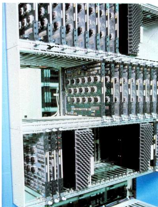
View of a System 12 cabinet with the doors removed showing some of the printed boards in the Aarhus exchange.
