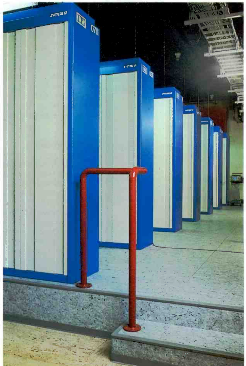
System 12 local-transit exchange installed at Aarhus.
