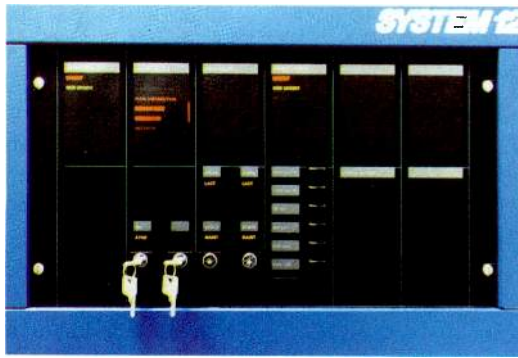
Main alarm panel for System 12 maintenance.
