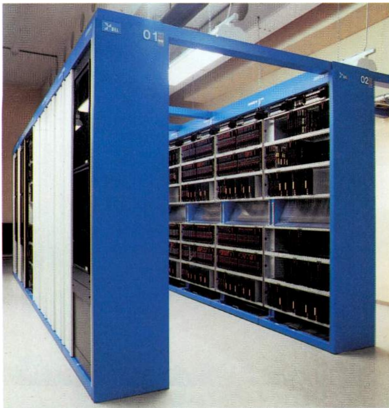
Small 800-trunk System 12 exchange in Heilbronn.
