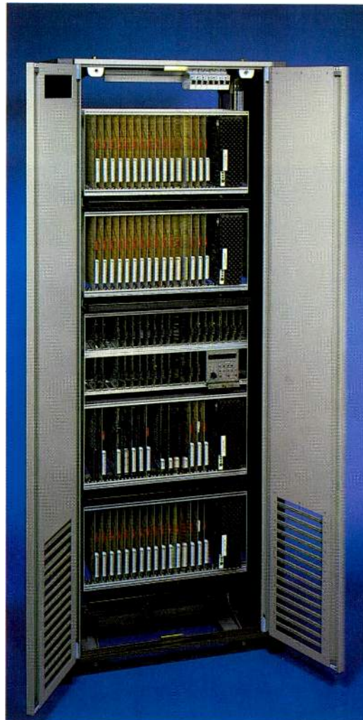
ITT 5500 business communication system cabinet with the doors open to show the equipped subracks.
