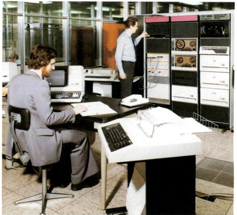
Processor and peripheral devices in an ITT 1290 operations and maintenance center.
