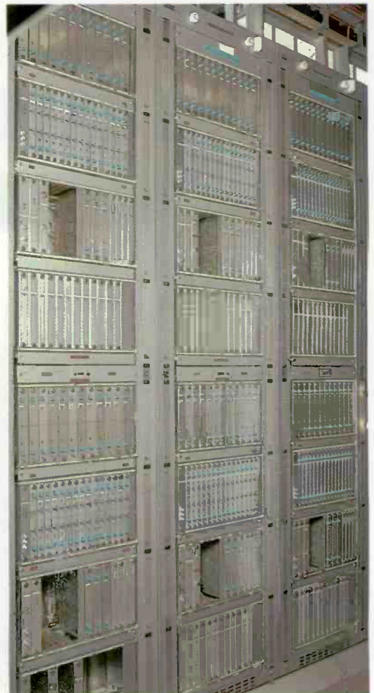
Unlink signaling converter, manufactured by NSEM, which overcomes the problem of Incompatible Interexchange signaling systems.
