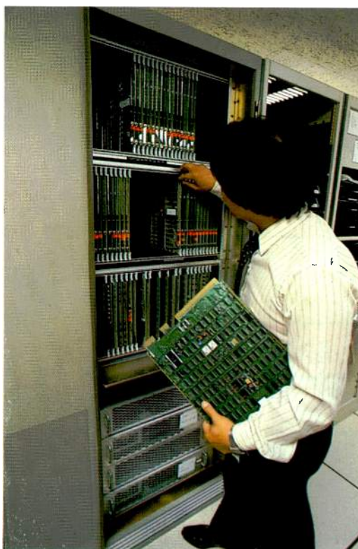
A view of the front end processor used for the Faxpak service. This provides all the necessary compatibility conversion between dissimilar facsimile terminals.
