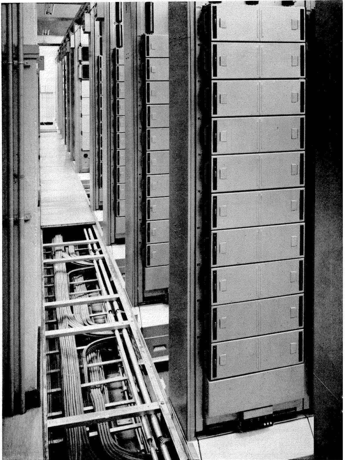
Figure 14—Cable run on switch-room floor at end of switch-rack rows.
