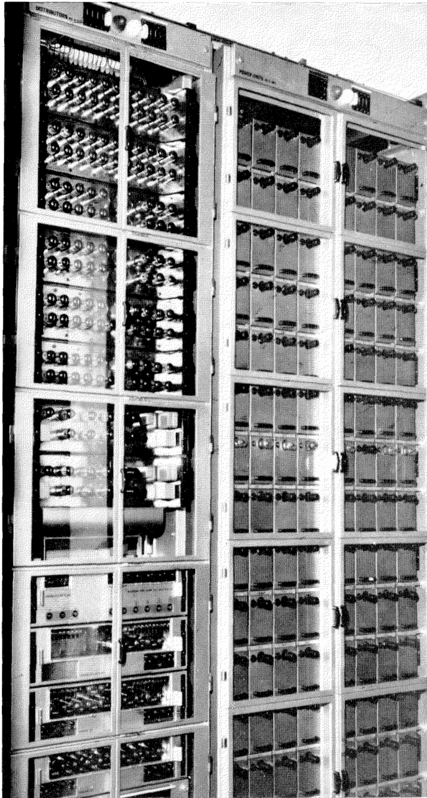
These two of the three bays house the pilots, distributors, amplifiers, and control circuits.
