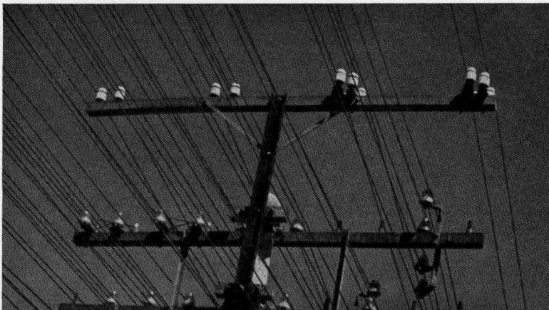
Figure 12—Typical crossarms, insulators, and transposition brackets. The zero crossarm carries 5.9-inch (15-centimeter) spaced wires on type-2 porcelain insulators mounted on H-15 -type transposition brackets. The first crossarm supports wires with 11.8-inch (30-centimeter) spacings; they are carried on double-peticoat alkaline-glass insulators mounted on both point- and drop-type transposition brackets.
