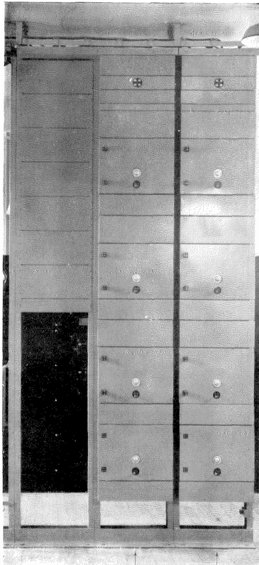
System 1-3 and spare amplifier.
