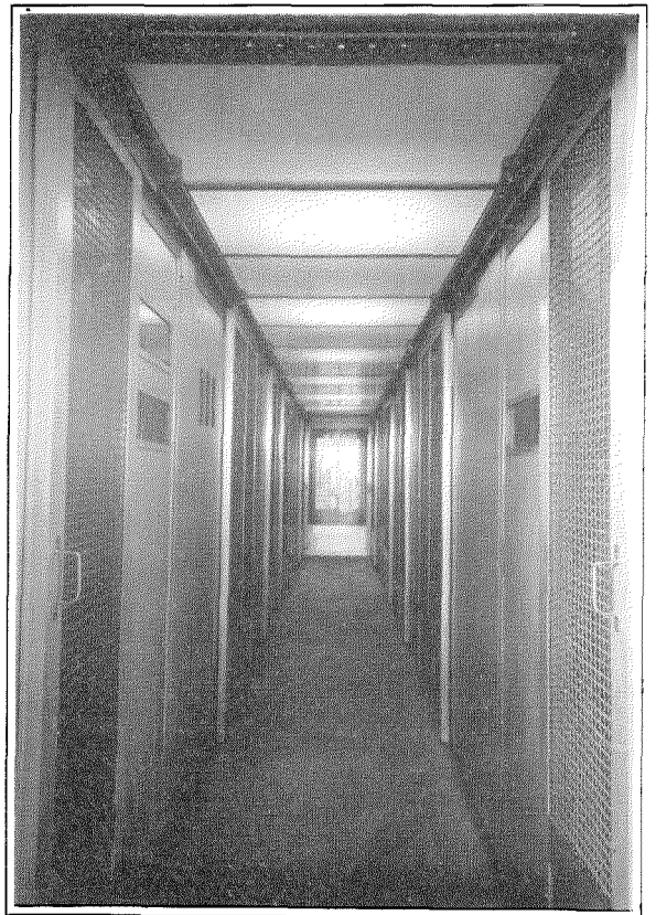
Fig. 6—Corridor of Cubicle Assembly.
