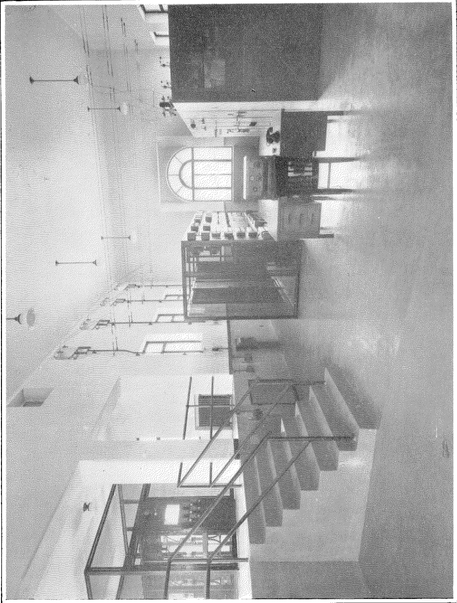
Transmitter Room at Hurlingham, Buenos Aires-New York Circuit
