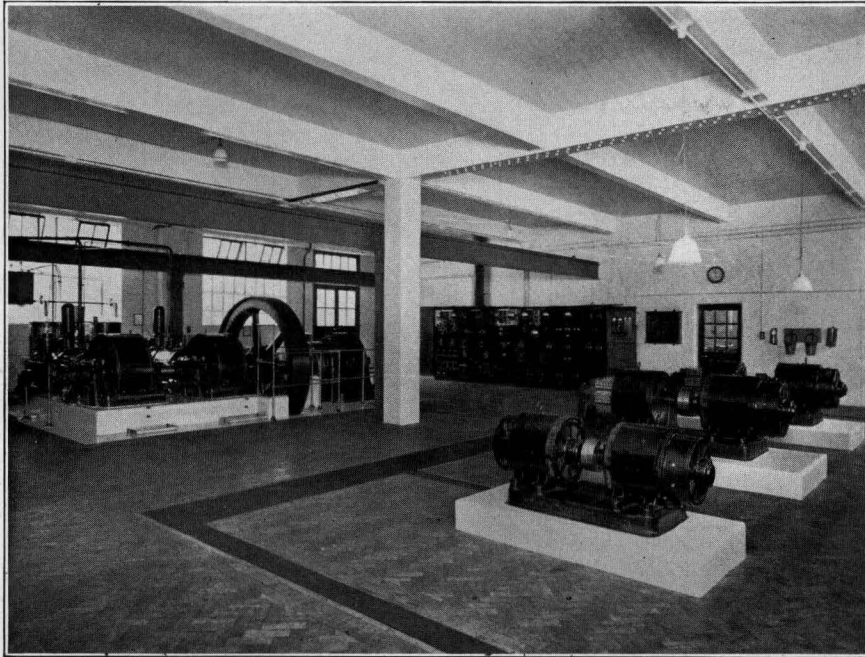
General View. Power Room, Derby
