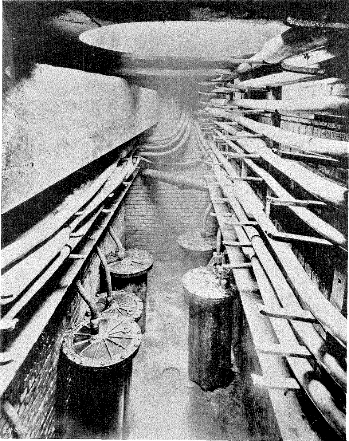
Figure 11—Loading Coil Cases Installed in Underground Vault
