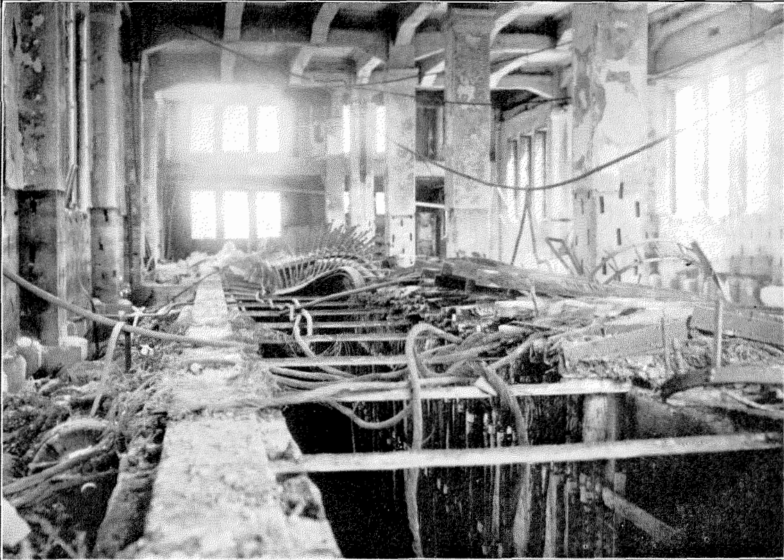
Figure 16—Ruins of M. D. F. and Office Manhole After Fire in Telephone Central Ginza, Tokio
