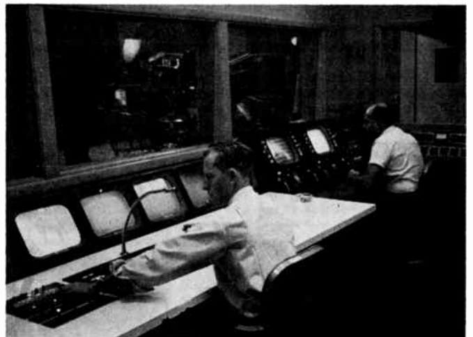
Fig. 2—View of a typical control booth for a television studio, showing program director's position, video control center, and audio controls. (Photo courtesy of South Carolina ETV Center.)
