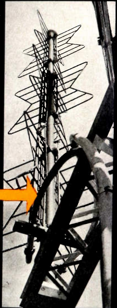
Typical TV antenna installation of Styroflex coaxial cable as a power line from station transmitter to antenna.
