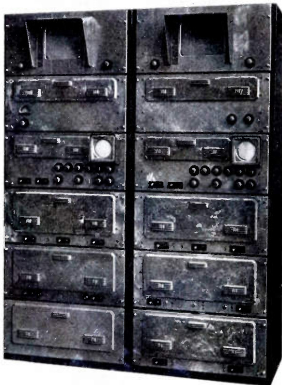
Fig. 8—Control racks of the relay.
