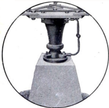
Base insulated central pier showing "Mast-Base" or "Pivot" type base insulator with Spark-Gap.
