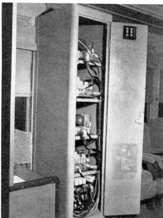
Fig. 9—Radio equipment installed on train.
