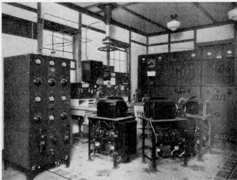
Fig. 1—Interior of aeronautical radio station at Glendale, Calif.
