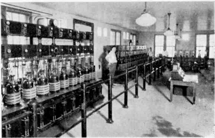
Fig. 12—Transmitting apparatus at station WEAJ.
