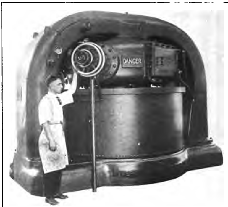
FIGURE 39—1,000-Kilowatt Arc Converter (Cathode Side)
