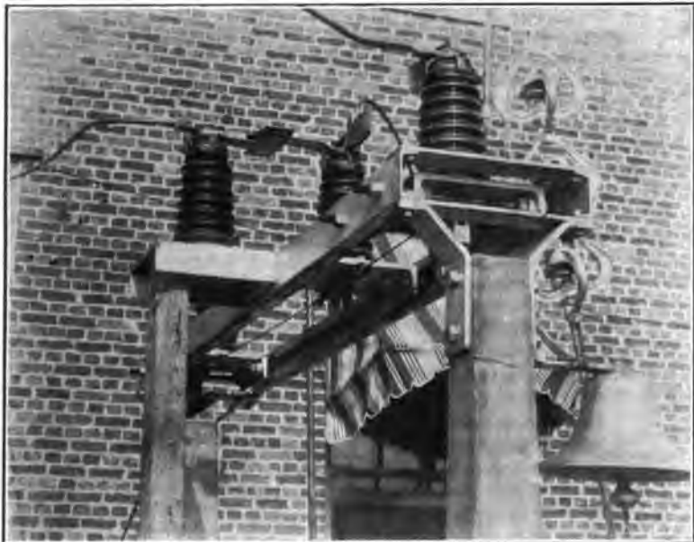
FIGURE 8—Antenna Switch, Arlington
