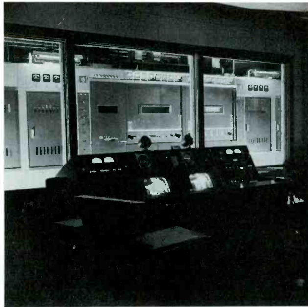
Fig. 5. KMOX-TV control room.
