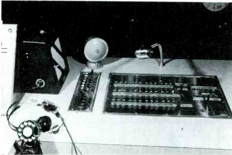
Fig. 3 - Photograph showing location of turret relative to the video switching panel at the TD position.
