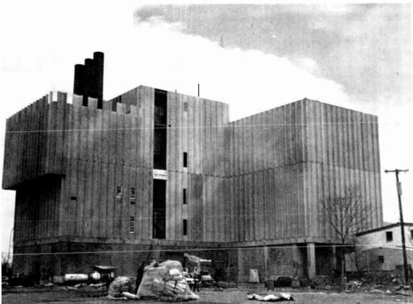
[1] This incinerator facility under construction in Nashville, Tenn., generates steam which will provide year-round heat or air conditioning to nearby government office buildings.
