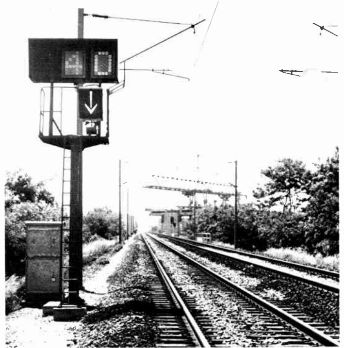
[2] Downward arrow, or "fleche," indicates to the train operator on the French National Railways that a decrease in speed must be made to the indicated 40 km/h. This indication is made automatically from a computer-controlled tower system.
