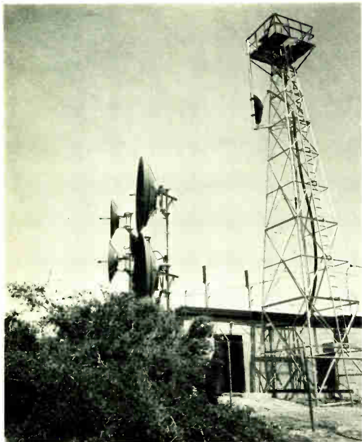
FIGURE 6. Black Mountain transmitter facility. Semi-omnidirectional antennas are mounted on the tower; directional antennas are mounted on pipes attached to the transmitter building foundation.
