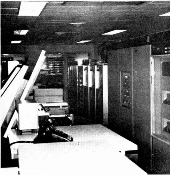
FIGURE 1. The "heart" of The Washington Star's automated capabilities—the central computer and data-processing center—containing two IBM 1800 computers, a Honeywell 200, and an IBM 1401.
