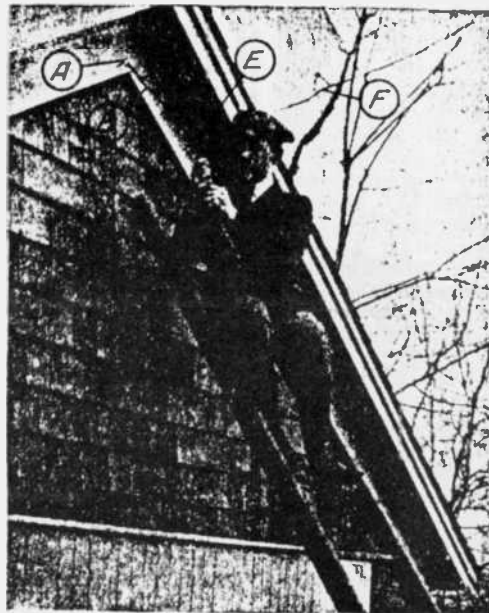
II Fastening the far end of the antenna through the metal eye of the insulator. A is the screw eye, B a piece of rope, the insulator and F the antenna wire.
