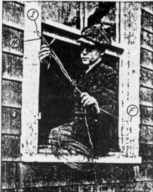
I Fastening the insulated lead in wire to the antenna wire. F is the antenna wire, G is the insulator; H is a piece of rope, I a screw eye and J the lead in wire.
