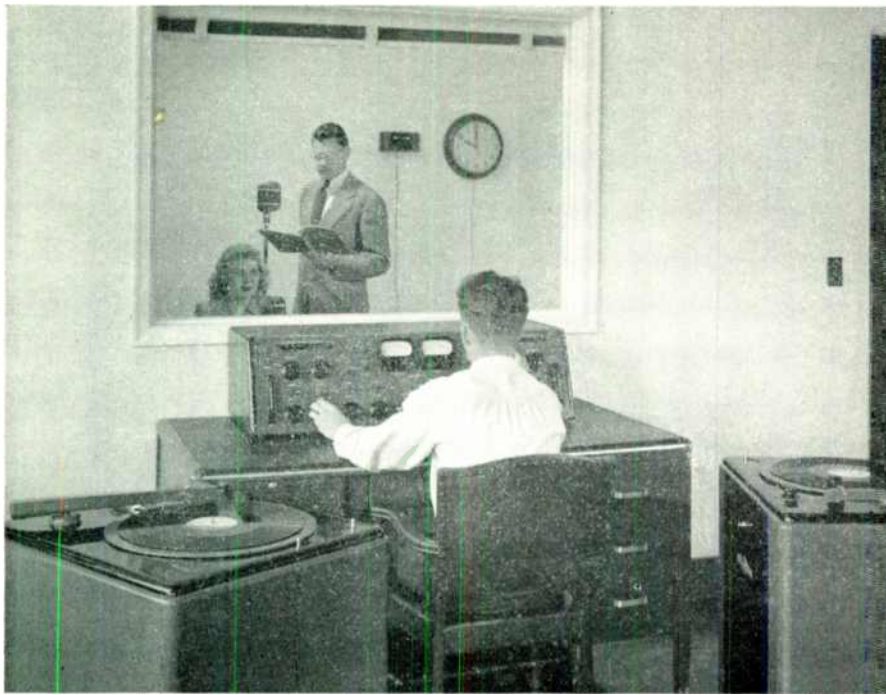
FIG. 15. Here is a typical control room setup for an FM or AM station of moderate size. There is a second studio at the left, and an announce booth at the right
