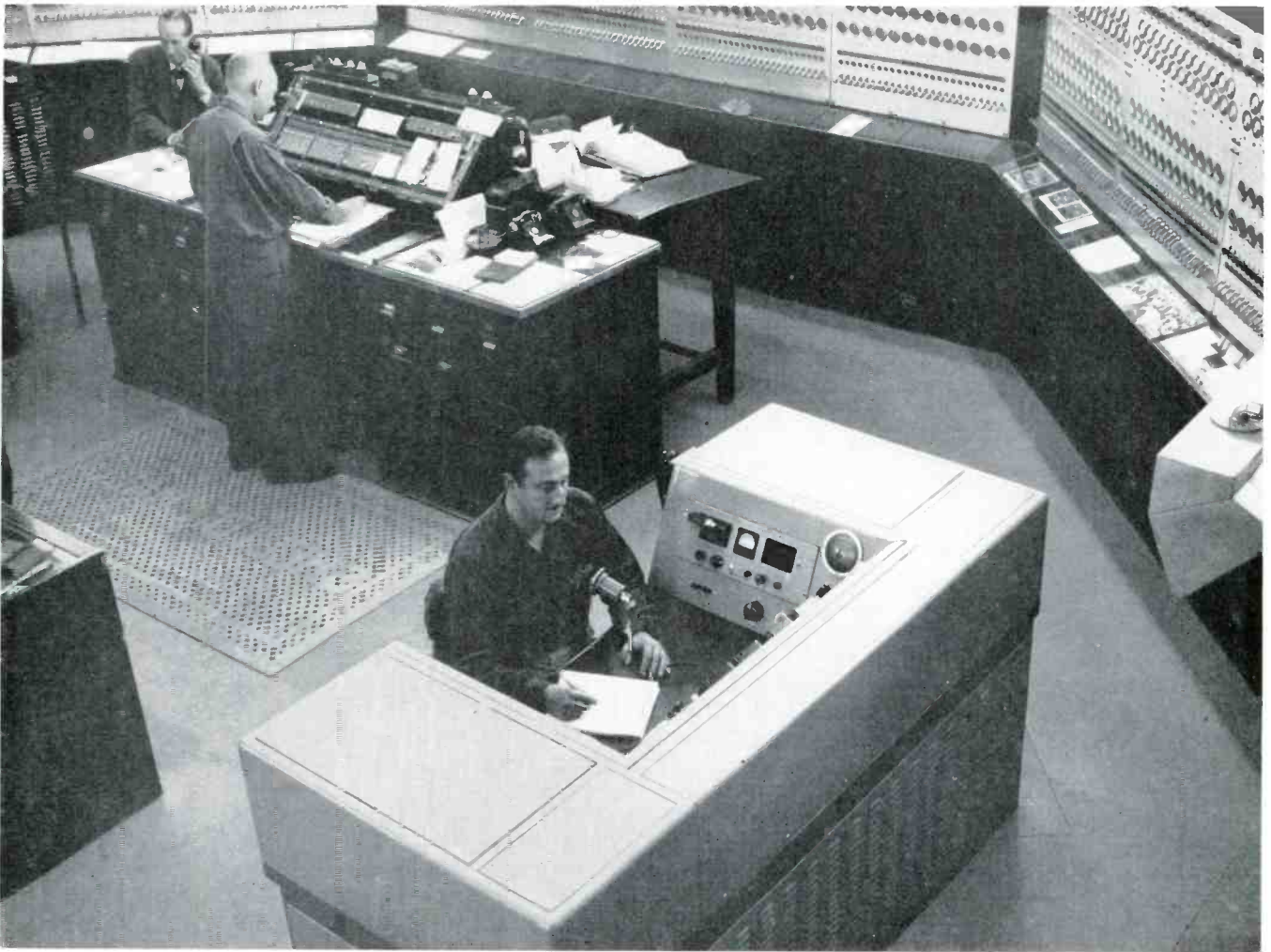
FIG. 1. CONTROL CONSOLE IN THE QUEENS FIRE ALARM CENTRAL OFFICE. BOTH BROOKLYN AND QUEENS TRANSMITTERS CAN BE CONTROLLED FROM HERE
