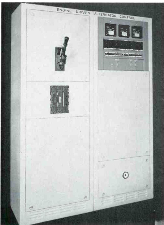
FIG. 4. A WESTERN CONTROL PANEL FOR TWO ENGINE-DRIVEN GENERATORS
