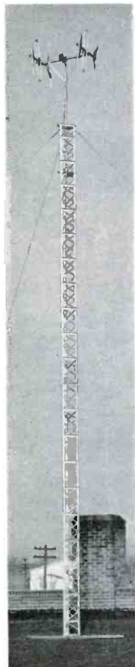
LEFT: ALPRODCO TOWERS ARE USED AT THE SHOPS AND OTHER REMOTE CONTROL POINTS
