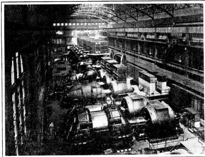
The largest electric railway power house in the world is located in the heart of New York City
