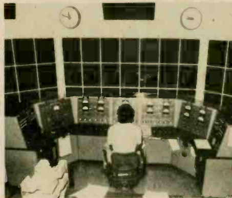
Transmitter control room technician adjusting equipment of the Okinawa relay station, Voice of America Radio, Ryukyu Islands
