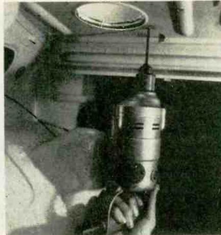
Fig. 7. Here's how it looks from inside the trunk. Note that in this car even the speaker mounting holes are pre-punched. Just drill through the rear deck cover from the trunk side. The metal tabs at the rear hold the speaker wires when they are bent upwards.
