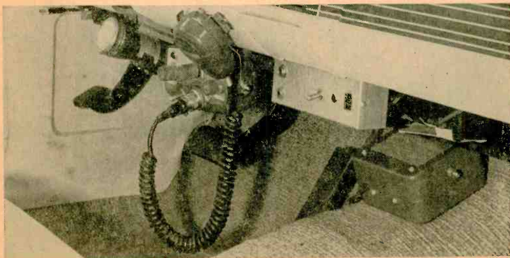
Completed mobile power station packs plenty of electrical convenience into small space under dash. Both 12 VDC and 117 VAC are available for powering wide variety of electrical accessories and experiments.
