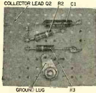
Only three components appear on bottom of perf-board: capacitor C1 and resistors R2 and R3. Collector lead from Q2 (see call-out) runs to one side of lamp I1; screw holding ground lug in place also supports perf-board mounting bracket (see photo at left),
