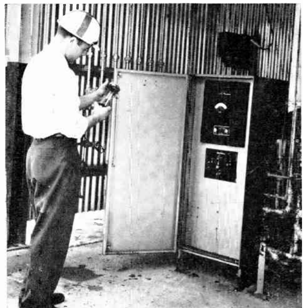
Engineer spot-checks oxygen analyzer
