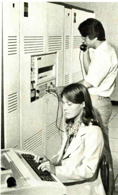
New switch. Phone company employees monitor operation of Stromberg-Carlson digital switch, first in nation to be installed in small, local telephone exchange.
