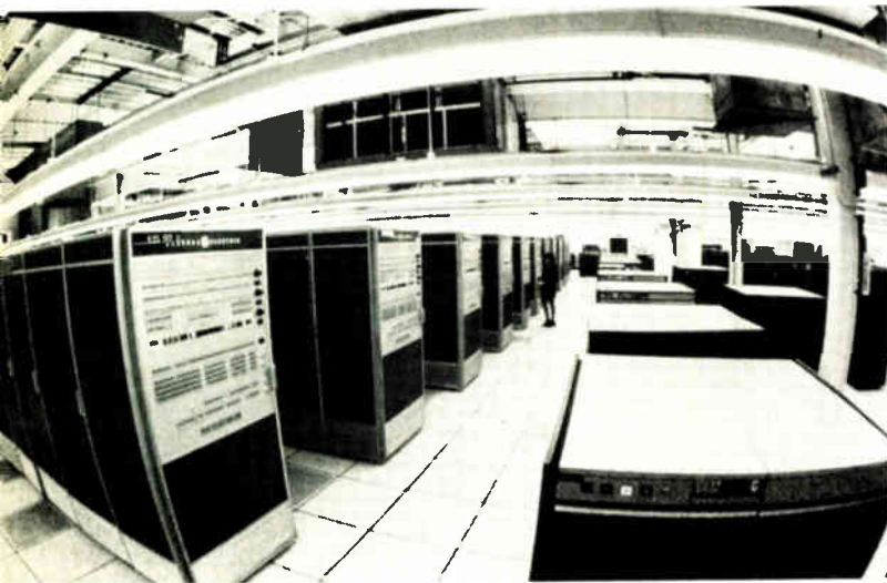
3. Network center. Large-scale Honeywell computers in Cleveland, Ohio, constitute the 15 foreground and two background computers to which the world-wide GE network is connected.
