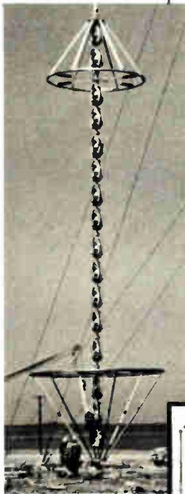
Large structural-guy insulator assembly with grading rings
